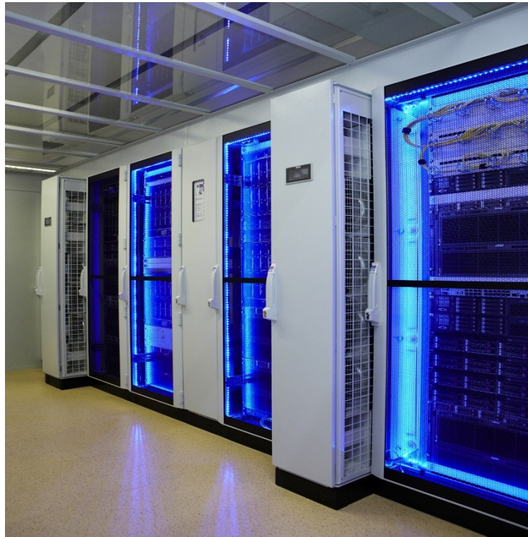
Fig.16. An approximate appearance of the LHEP off-line cluster-216.
